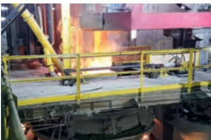
The electrics and automation system of the Presidente Vargas plant was modernized.
