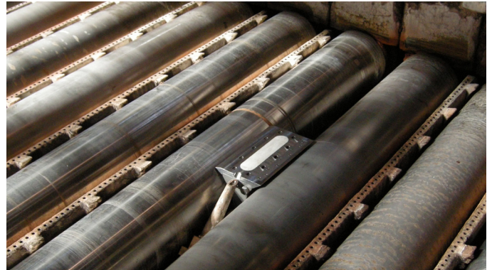
Transformation Monitor installed in the mill
